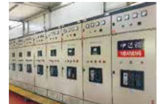
synchronization cabinet parallel cabinet 并网并网柜
